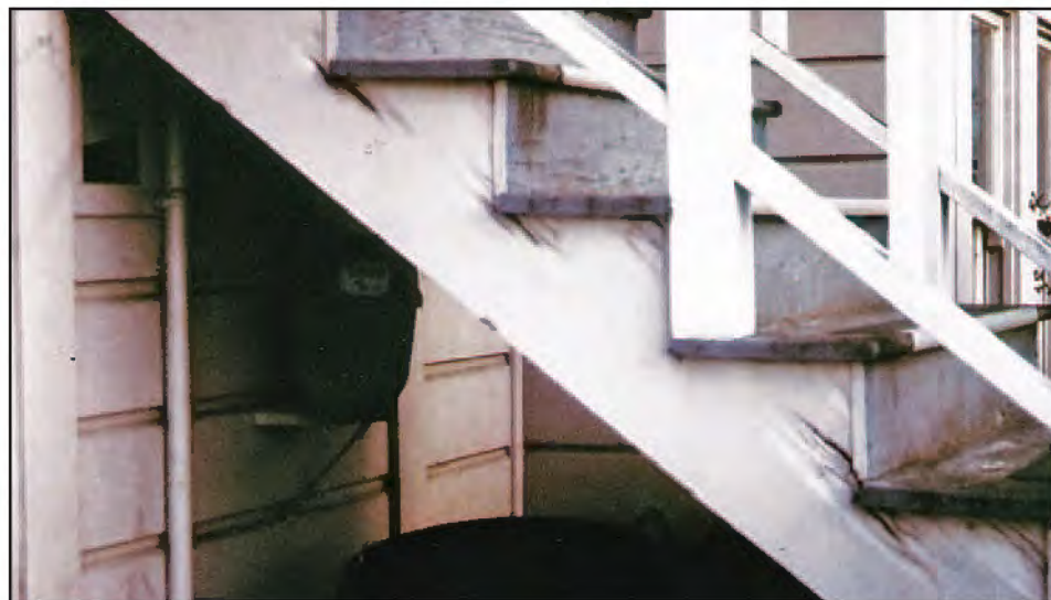
Figure 13-13. Deterioration in a notched stair stringer
