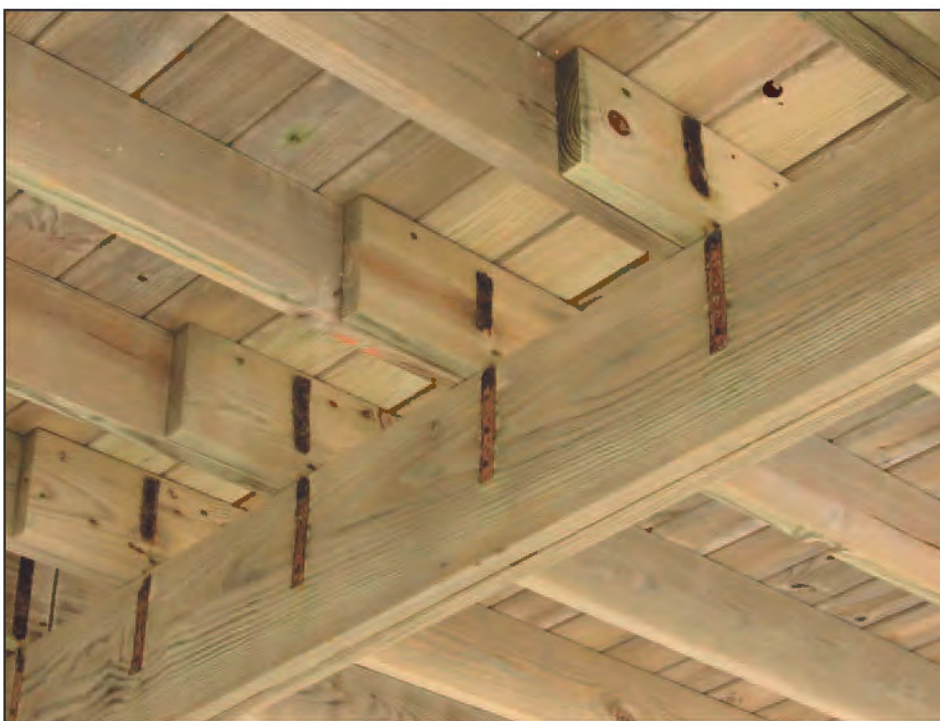
Figure 14-3. Severely corroded deck connectors
