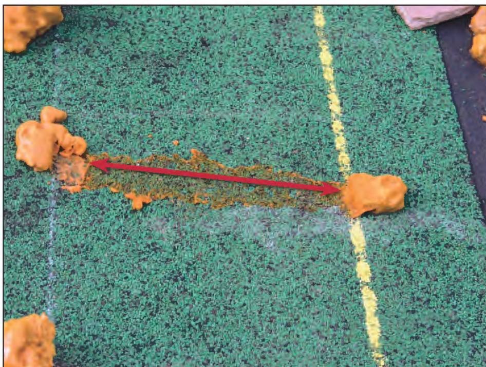
Figure 11-44. Adhesive that debonded from the cap sheet
