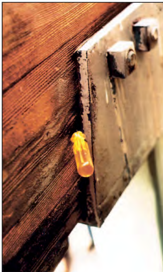
Figure 14-2. Wood decay behind a metal beam connector
