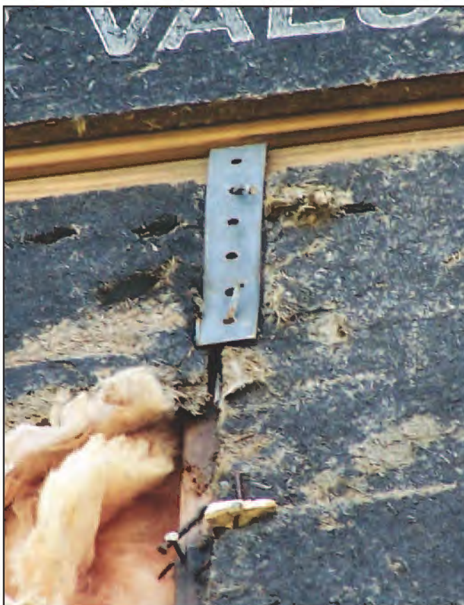
Figure 13-15. Connector failure caused by insufficient nailing
