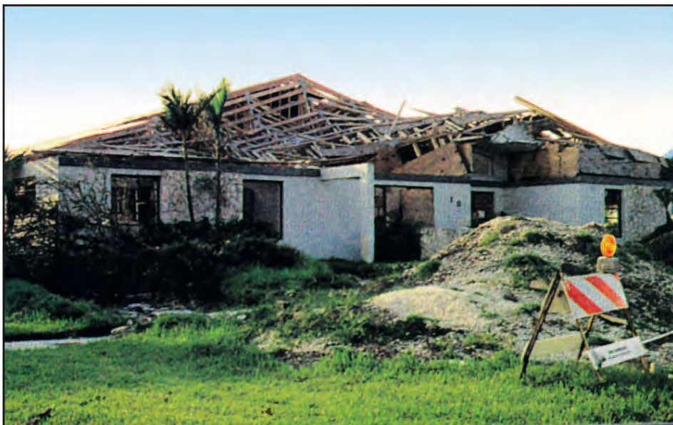
Figure 9-21. Gable-end failure, Hurricane Andrew (Dade County, FL, 1992)
